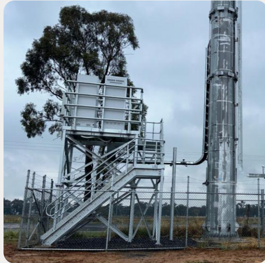
The Gooloogong Fixed Wireless Site (NSW) was elevated in December 2023 after sustaining extensive flood damage in 2022
